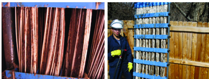
Figure 7. Hollow-fiber membranes after a sludging episode (left). Operator cleaning sludged membranes (right).
