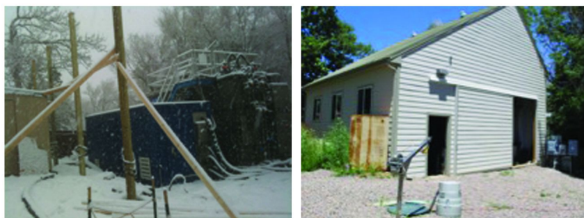
Figure 6. SBMBR before (left) and after (right) the construction of the weather protection structure.
